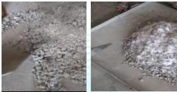
Figure 2: steel and polypropylene fibers mixing with aggregates & cement before adding water to mix
